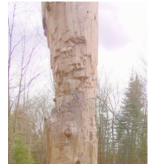
Figure 6: Wood pole damaged by a bear.
