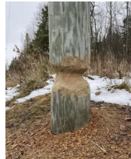
Figure 5: Wood pole damaged by a beaver.
