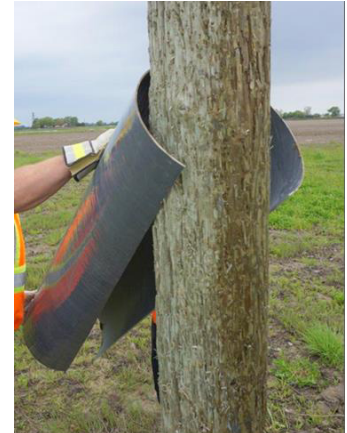
Figure 10: Spreading the primary shield while pushing inward and upward onto the destination pole.
